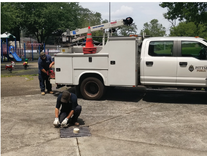
Pittsburgh Public Works Ironworker Mike (kneeling) secures grating as laborer Rich prepares hardware for repairs to the Marmaduke Park spray feature on June 15, 2020.
